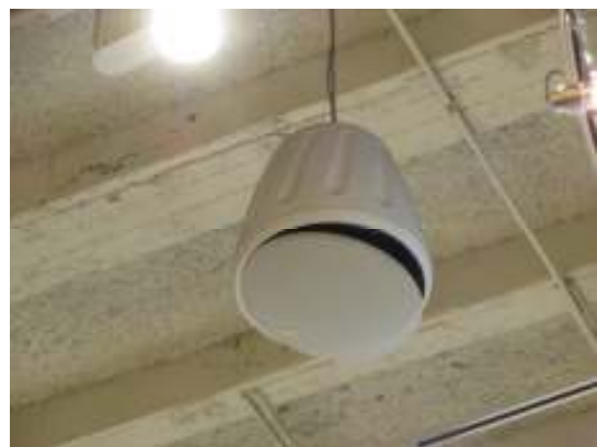
Store overhead speaker cover at risk of falling
