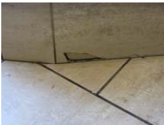
Damaged store wall tile near entry doors
