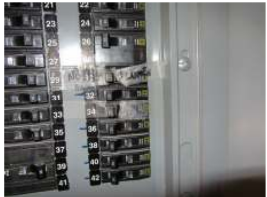
Improperly taped circuit breakers
