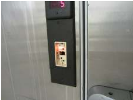
Damaged freezer control panel
